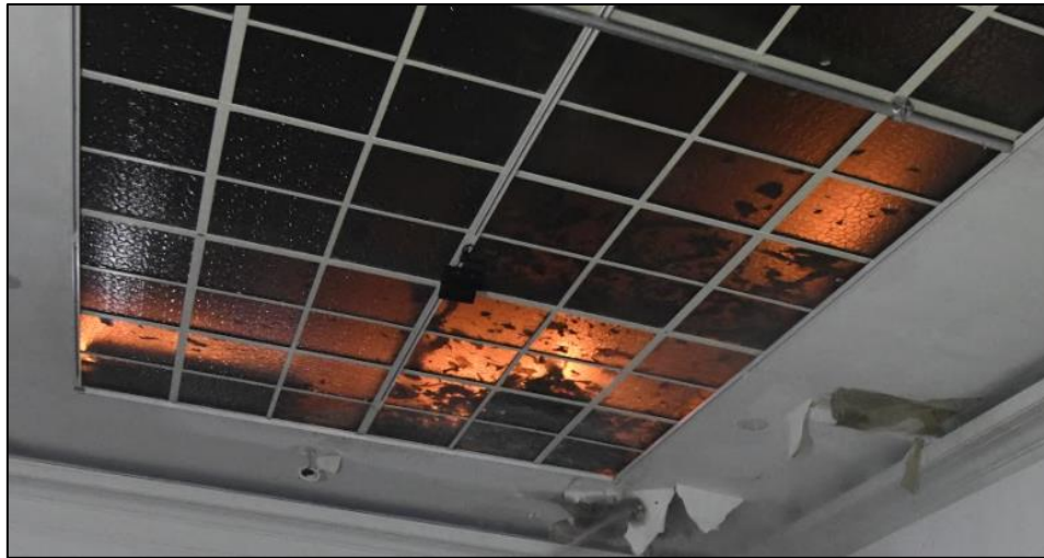
Image 7 View at a glass section of the false ceiling. The fire in it is clearly visible. (Picture: Luc Van Ussel)
