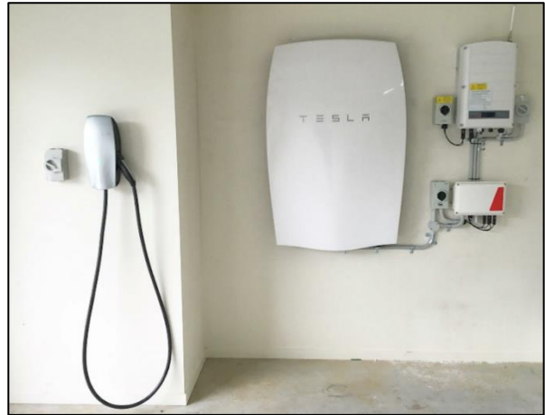
figuur 4 Tesla brings a number of applications on the market to store large quantities of electricity. The fire behavior of these devices will probably be problematic in the same way as the fire behavior of the batteries of electric vehicles. (Picture: www.mcelectrical.com.au )
