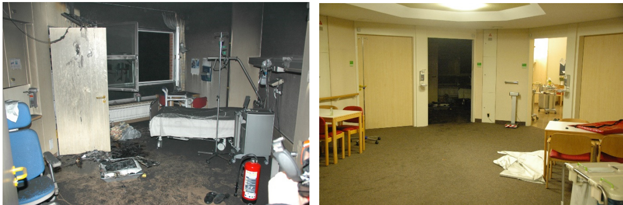
Figure 9 Fire in a hospital room in Germany. The left picture shows that the hospital room was completely smoke filled. The right picture shows the hallway. In the middle of the picture is the door leading into the fire room. There is no smoke damage in the hallway. The smoke stopper is on the floor at the right end of the picture. (Photo: Michael Reick)
