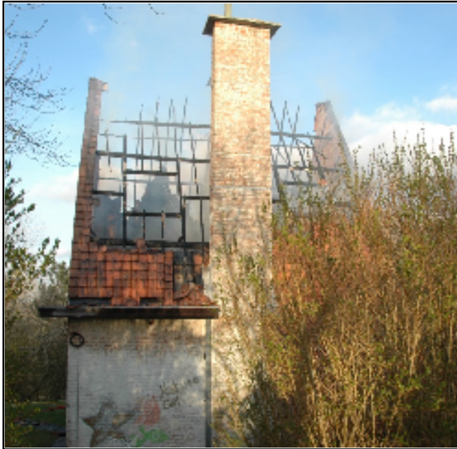
Figure 1 The fixation points of the bales have been partially burnt through. When wind conditions are fierce, these gables may collapse. The chimney is probably attached to the rafters as well. There may be damage at this point also. (Photo: unknown)
