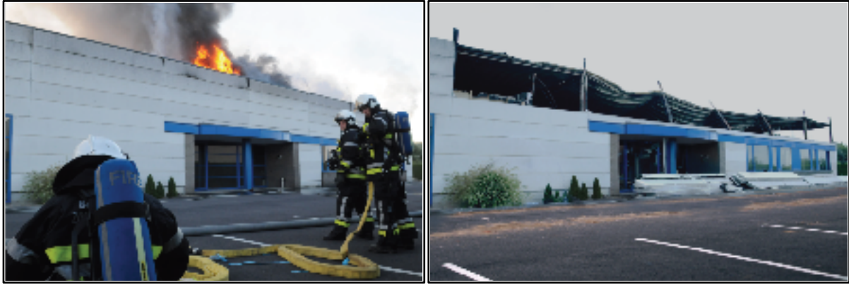
Figure 4 A fire in an industrial building made up out of prefab wall panels. Because of the risk for collapse, distance to the wall is kept. Afterwards, any loose panels are removed to eliminate the any risk for collapse. (Photo's: Peter Vangierdegom)
