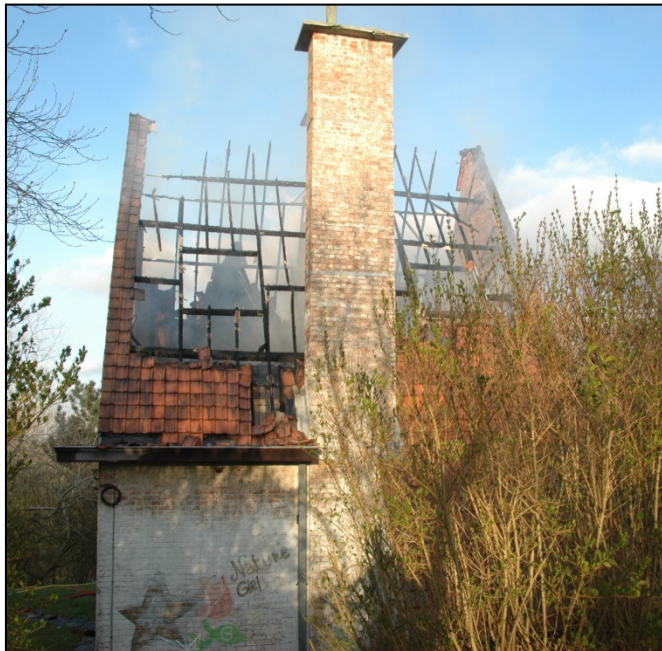
Figure 1 The fixation points of the bales have been partially burnt through. When wind conditions are fierce, these gables may collapse. The chimney is probably attached to the rafters as well. There may be damage at this point also. (Photo: unknown)
