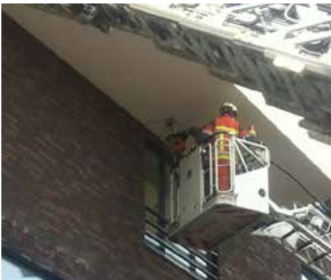
The crew moves five meters and makes a new cut. Photo by Pieter Maes
