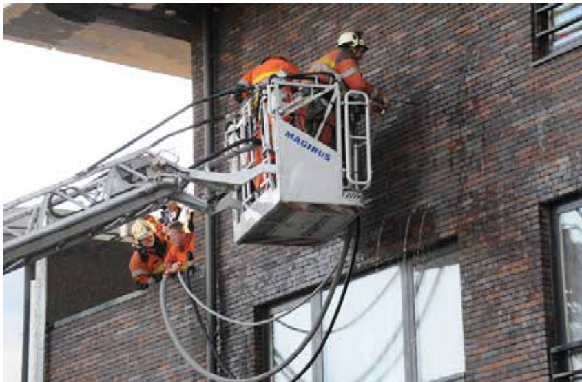
Piercing nozzles in use. First a hole was made using a power drill. Next a piercing nozzle was used to flow water inside. The water was running downward over/through the insulation.
