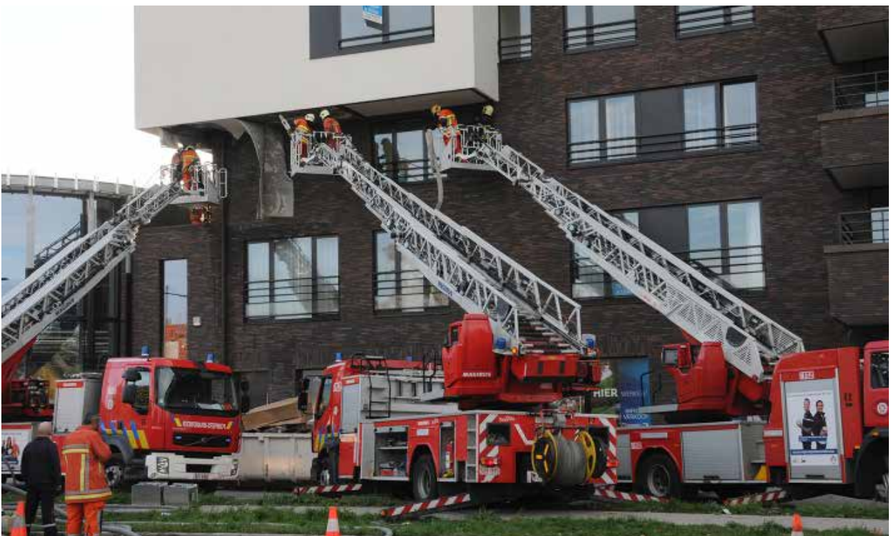
Three ladder trucks working to clear the plaster and the EPS insulation. Photo by Robert Dekock
